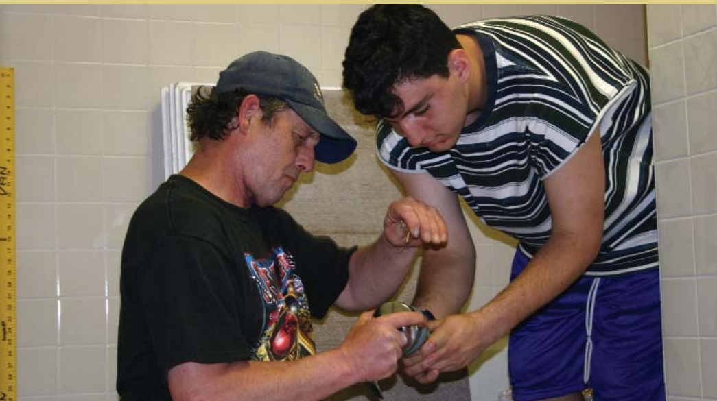
Larry Schiller (l) and Elvis Lynn put the finishing touch on the newly built handicap accessible bathroom at Vinfen's Employment Training Center, where they worked for four months.
